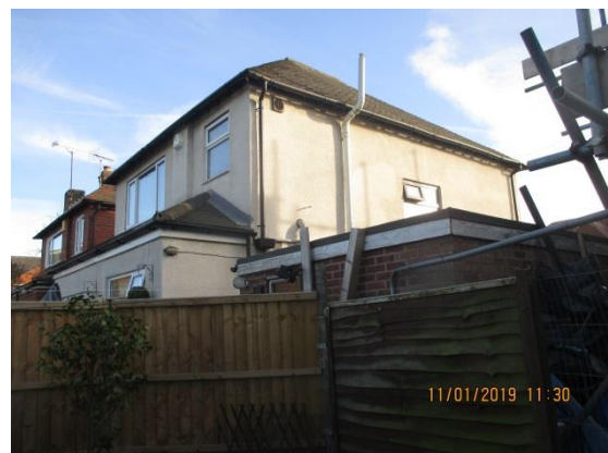
South west (side) elevation of application property from rear garden of no. 8 Muriel Road
